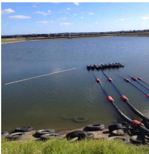
Dam extraction using submersible pumps to provide adequate flow for irrigation
