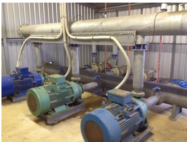
Pumps added in parallel to boost flow into the irrigation main
