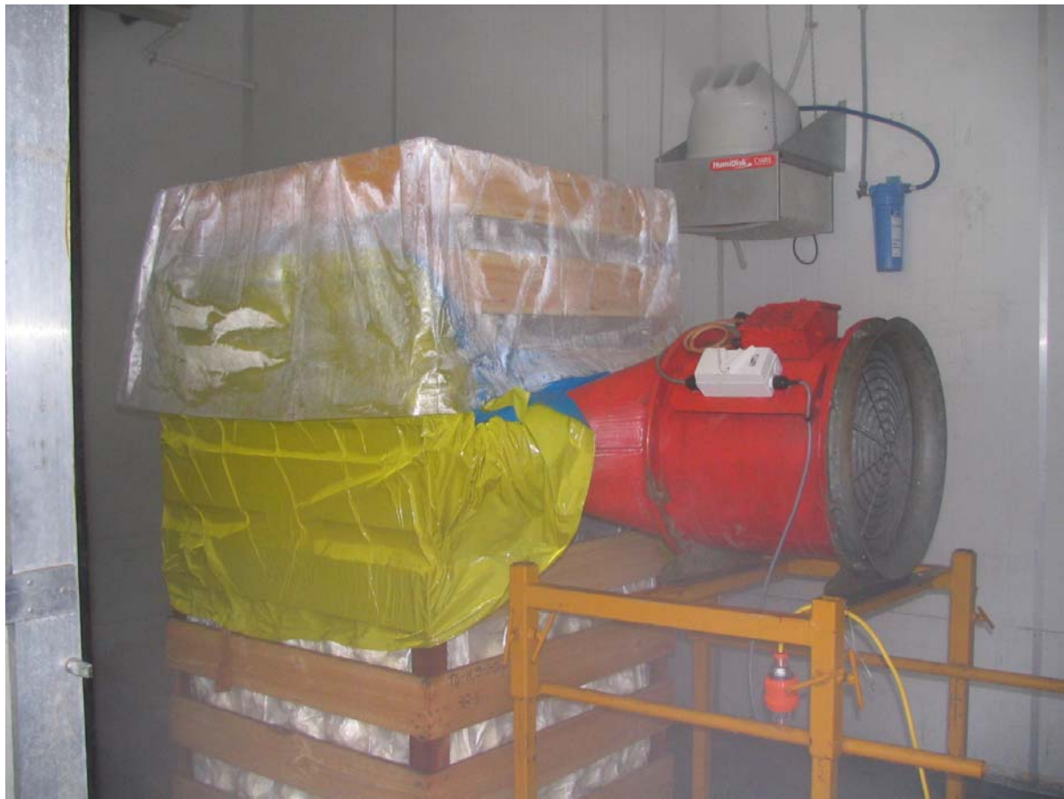
Figure 4.3. Pre cooling using an experimental portable fan and humidified air.
