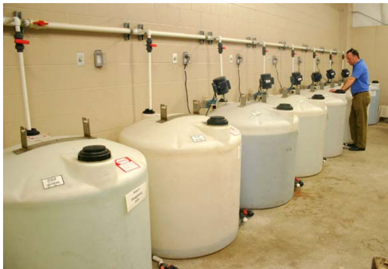
Tanks for holding the nutrient solutions. Some have small electric stirrers.
