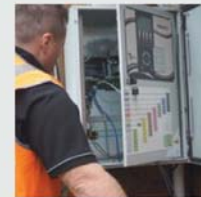
Installation of the Gateway which is used to communicate the data being captured by the sensors installed to the backend of The Yield solution. Data is uploaded every 15m. Once the trial is complete the Data Science team can complete the extraction process for conversion in the analytics.
