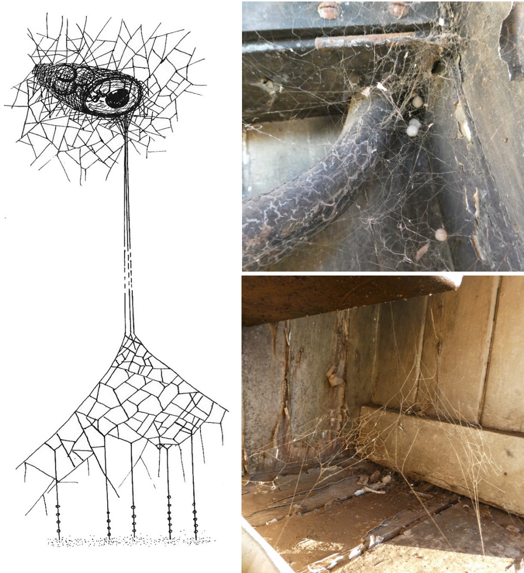
Figure 6. Typical structure of a redback spider web, from B York Main (left) and the retreat (top) and tangle web (below) typical of a redback living inside an electrical box on farm.
