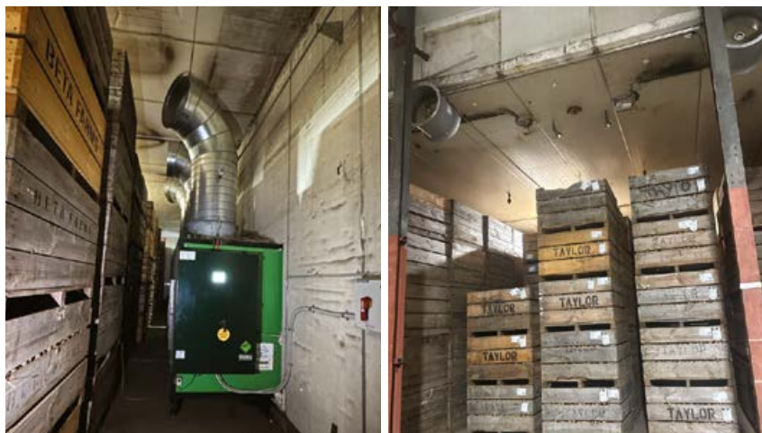
Figure 7. The Tolsma blowing ventilation system at Coldahold, WA uses large pipes to blow air through the room (left), with additional fans installed at intervals to ensure even distribution (right).
