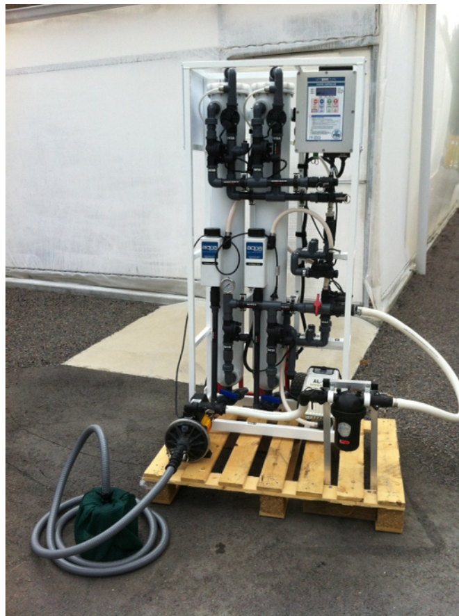
Figure 1: One of the ultrafiltration test units used in the research trials
